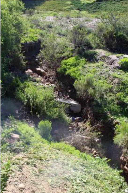
Incised channel created by unnatural erosion
